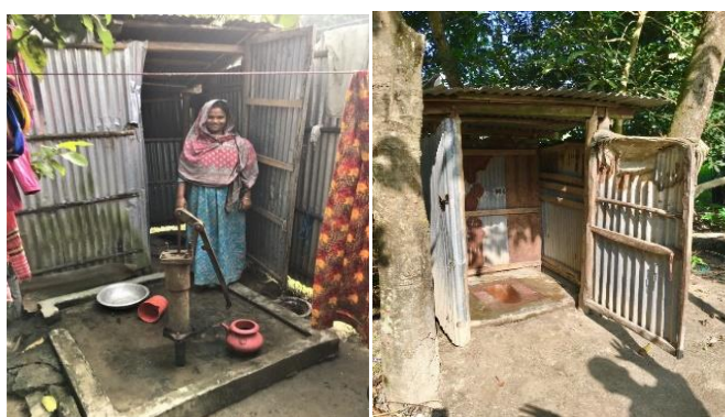
Examples of a newly constructed tube well and latrine in an ALO household during the project period
